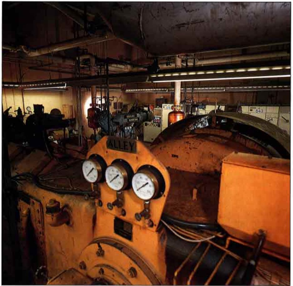
View across the compressor house
