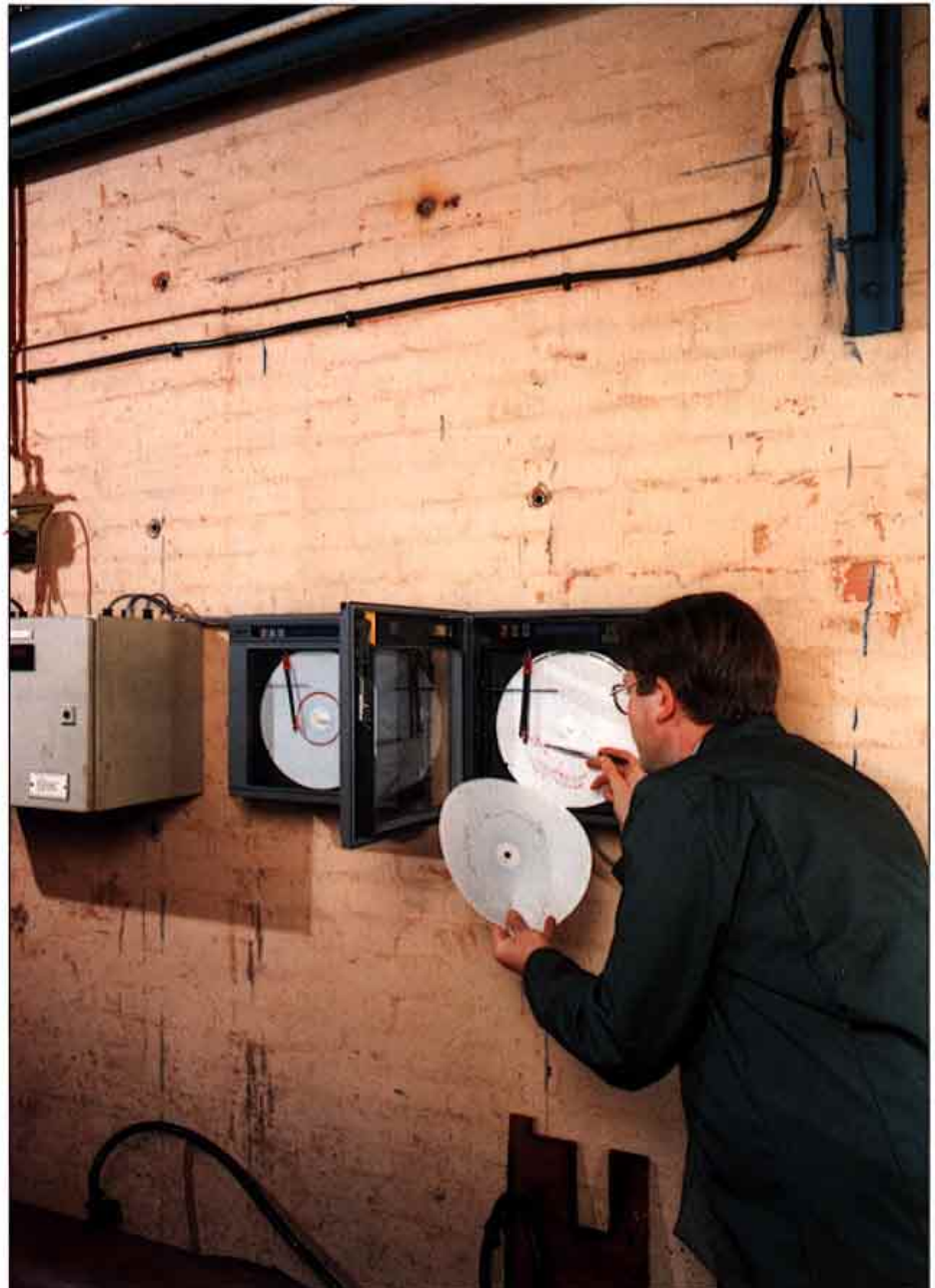
Checking the air flow and pressure record chart
