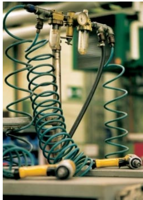
Fig. 3: Energy "gobblers" in compressed air system
